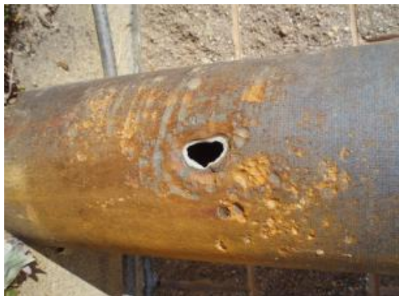
Fig. 1.4: Pitting corrosion of mild steel
