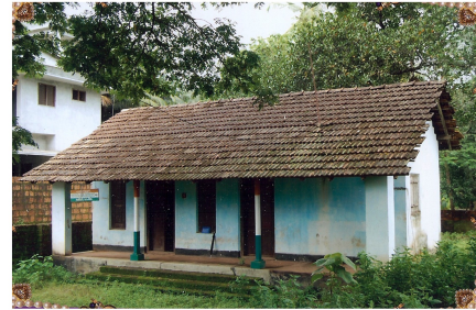
The Building of the Mahila Samajam (Pappinisseri) run by Gracy Aron, later donated to the Congress Party.
